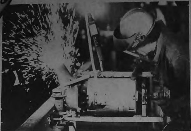
SPATTERING SPARKS —A worker grinds the newly-welded joint of two rails (Mark Wilson photo)
