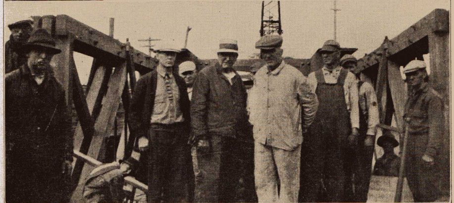
Upper —New span over Moose River, before removal of old structure. Lower —At work on Moose River Bridge. Bridge Foremen Coombs and Baird in center.
