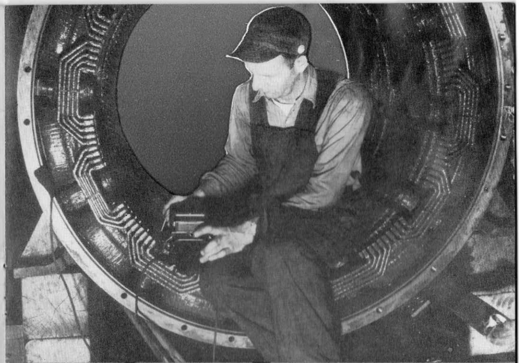
PUTTING a "megger" on a diesel generator at Waterville is Electrician Forrest Hussy
