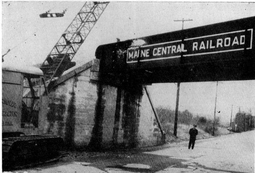
COMING DOWN at Rumford Junction is our overpass on the Portland-Lewiston Road. Bright spot above the "Maine" is burner's torch. Rioux Construction Company is doing the wrecking
