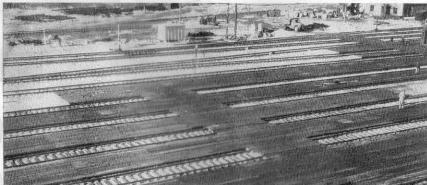
COINCIDENT with the rebuilding of the Union Station West Yard at Portland was the extension and rebuilding of the station platform with 75,000 board feet of treated southern pine
