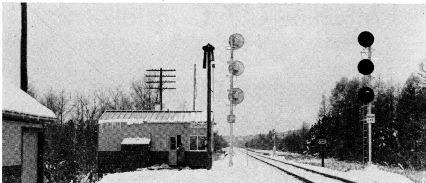
Tower MD with color light signals at East end of C.T.C. area. A temporary, manually operated train order signal stands close to the building while a permanent color light train order signal is being erected on the mast standing above the roof of the structure.
