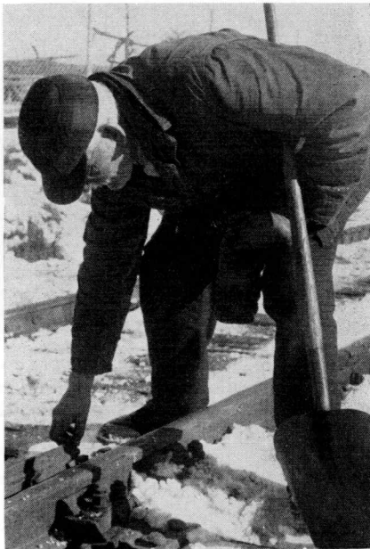
Close inspection of track and switches by Foreman McClure is part of his task to keep Section No. 191 in good condition.
