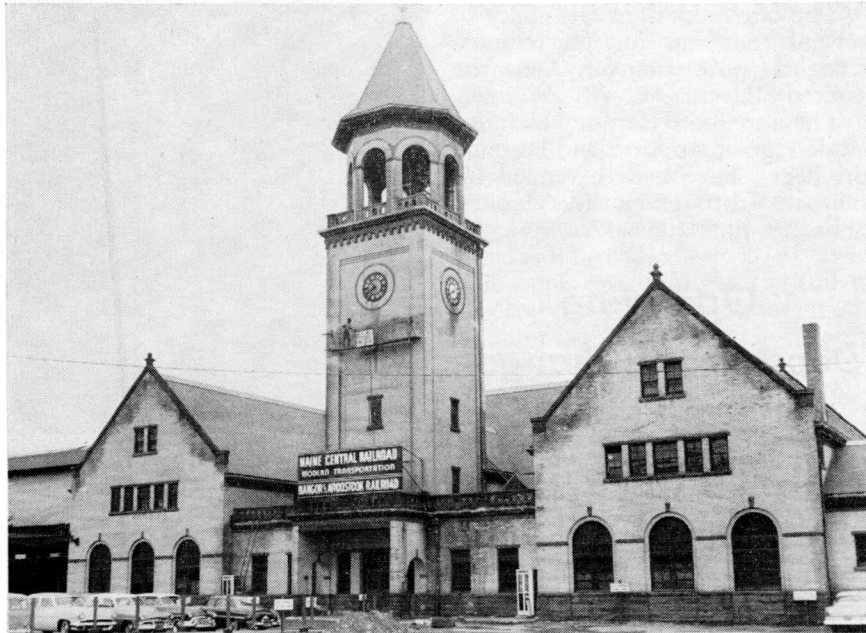
Steam cleaning of Bangor Station proceeds on the building's tower. Dirt, grime and stains made it hard going in spots.
