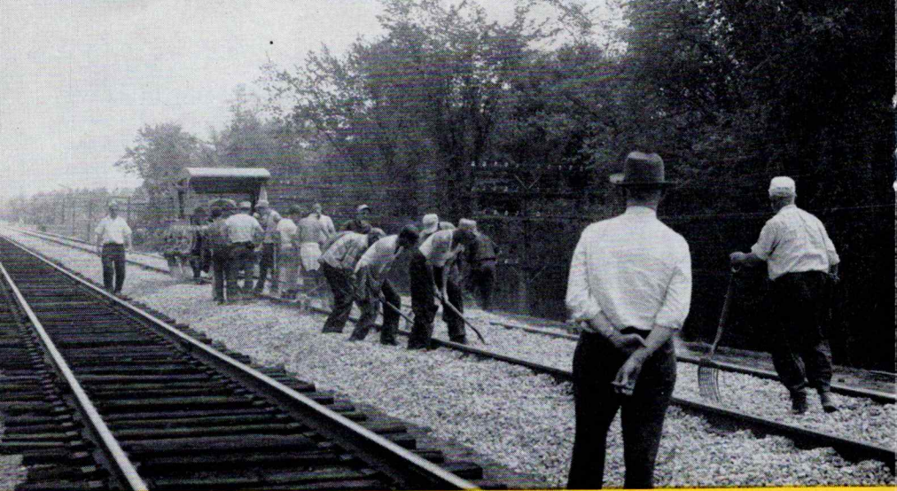
New crushed rock ballast was put in along the main line at Carmel as part of a busy summer schedule of track and roadbed improvements by our Engineering Department.
