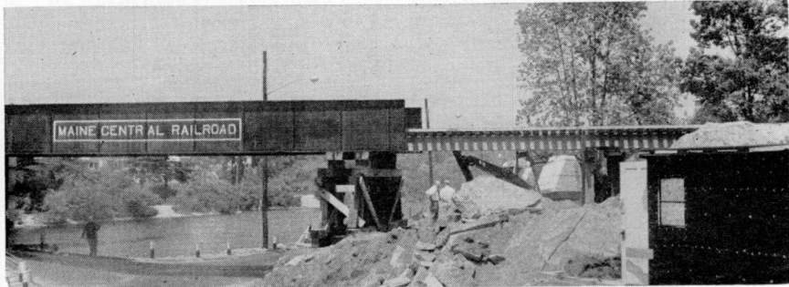
BEFORE—With the old 59-foot bridge section still in place, a temporary trestle lengthens it, to the right in this picture, while earth is removed and a new concrete abutment is constructed.
