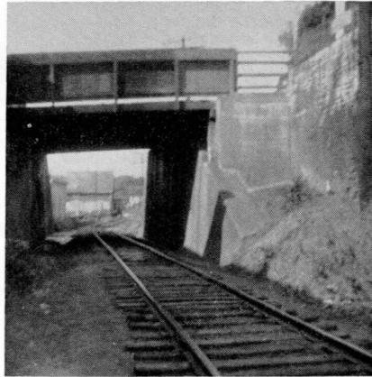
Note the smooth appearance of abutments of Main Street Overhead Bridge in Brewer following complete restoration of surface concrete.
