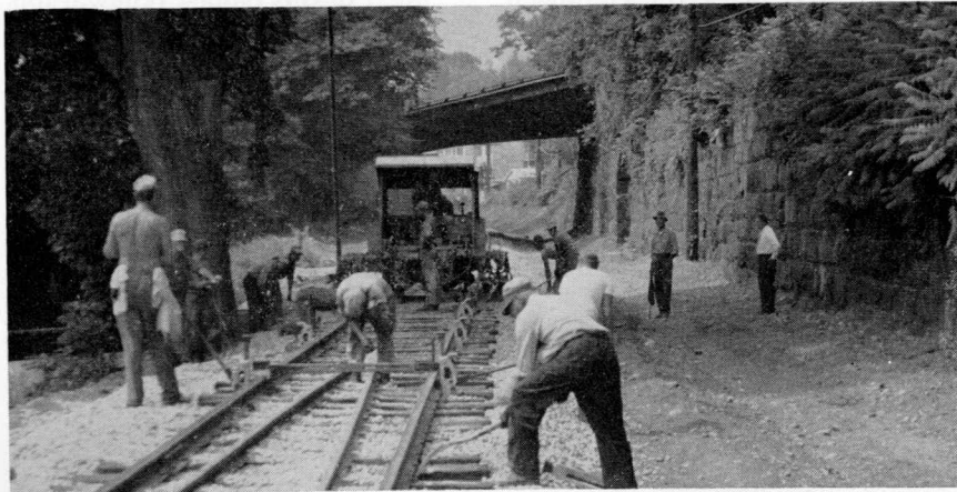
After a work train distributes crushed rock and track is raised to proper level, a Multiple Power Tamper seats the ballast beneath the ties. Standing at extreme right, is W. L. Harris, 3rd, Track Supervisor of Brunswick; second right is Earle Hamilton, Foreman, whose Extra Crew handled the work.
