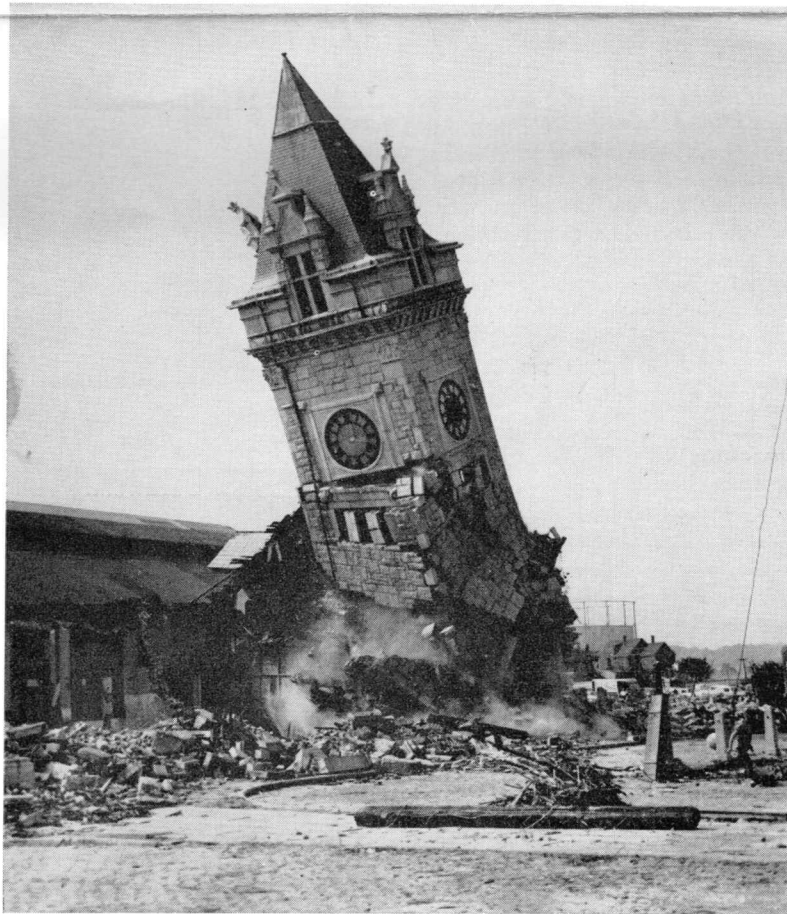
A LANDMARK FALLS —Historic Union Station Tower—a Portland landmark for more than three generations—crashed to the ground during demolition work in late August. This picture appeared in newspapers throughout the Nation. Construction of a huge shopping center on the site is expected to be completed in time for opening early in 1962.
