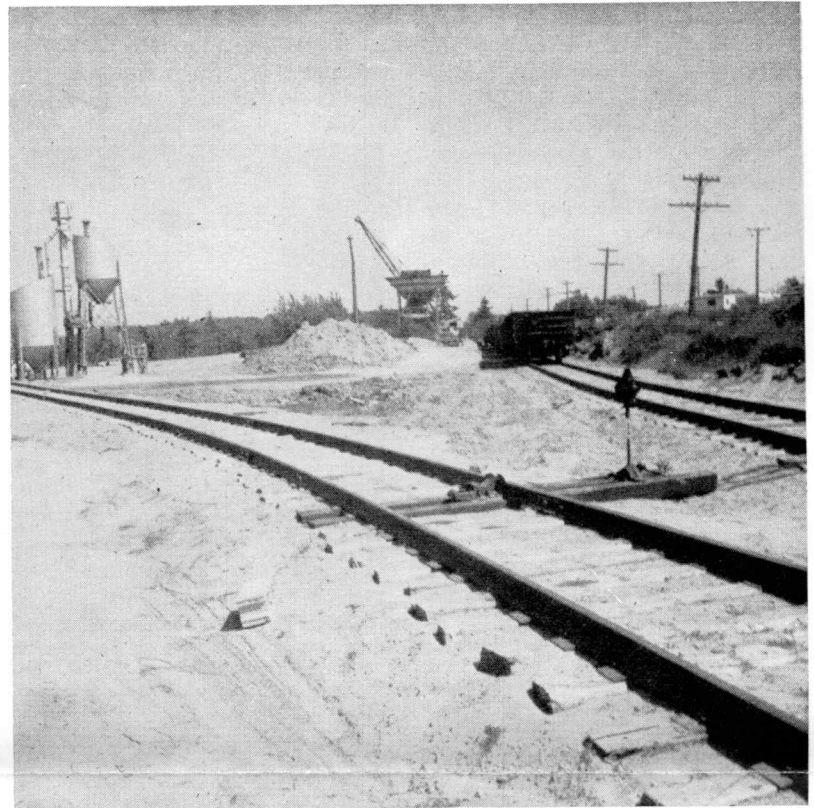
BUSY SPOT NEAR BRUNSWICK —This temporary installation at Cook's corner, near Brunswick, has served as a receiving point for 275 carloads of stone and 62 carloads of cement used in completion of a new highway project. The stone came from Leeds Jct., and the cement from the Dragon plant at Thomaston.
