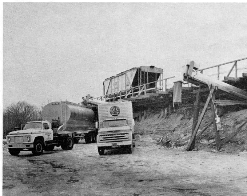
NEW UNLOADING FACILITY IN USE —Maine Central's new public unloading facility for bulk grain and feed in Auburn was used for the first time early in February. This is a Hales and Hunter shipment from Wilmington, Del., for the Roux Poultry Farm in Alfred. Other prospective users of the railroad-provided facility include Eastern States Farmers' Exchange, Maine Milling and Manufacturing Co., Beacon, Wirthmore, C. E. Thurston and sons, and several other grain and feed distributors in the Lewiston-Auburn area.
