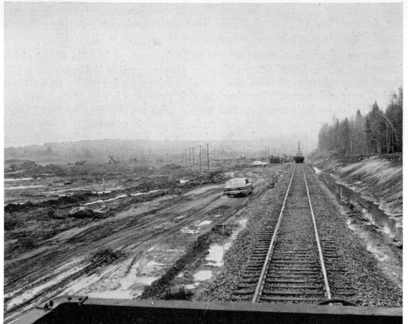
NEWEST STRETCH OF RAILROAD IN MAINE —This track is—or soon will be—the Rumford Branch of the Maine Central as it passes the site to be occupied by the new mill of the International Paper Company at Jay. This open area—about a mile long—has been cleared from the forest since mid-winter.
