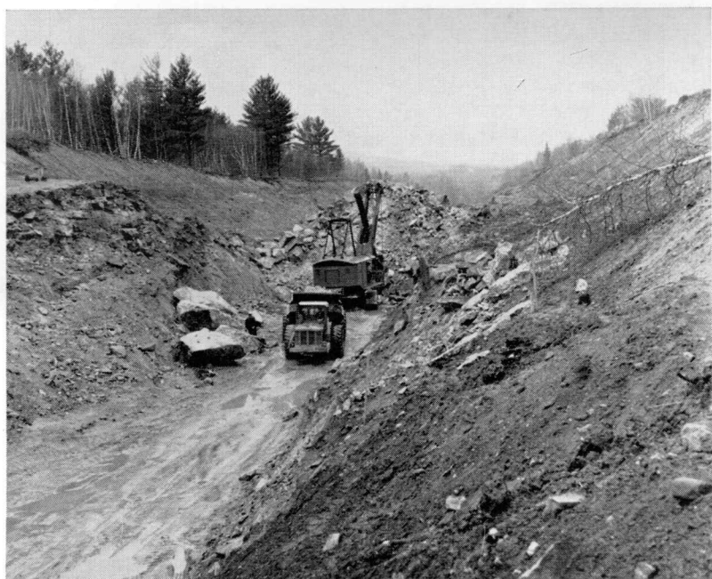
NEW CUT FOR RELOCATED BRANCH AT JAY —Men and machines are at work cutting away thousands of yards of rock and earth west of the site of the new International Paper Company mill at Jay for the re-located main line of the Rumford Branch.
