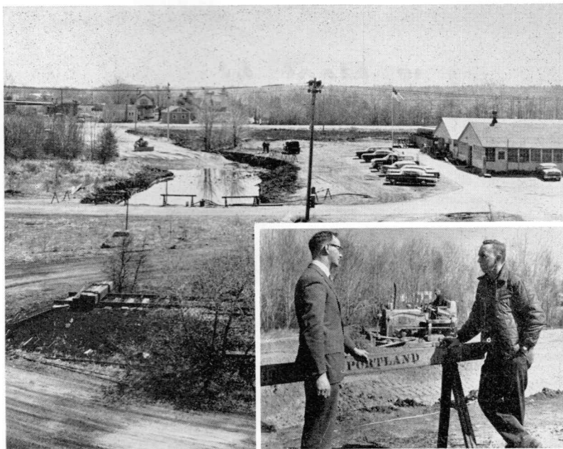
WILL IT BE "FLYNN STREET?" —The City of South Portland is building a new access road to the Rigby engine house and stores department area to eliminate the dangerous route One entrance. The new road runs from the entrance road from the nearby industrial park to the Stores Department buildings. Inset shows Hugh R. Flynn, Storekeeper at Rigby, who as a South Portland City Councilor urged construction of the new access road, discussing progress with Edgar Kierstead, street superintendent, City of South Portland.
