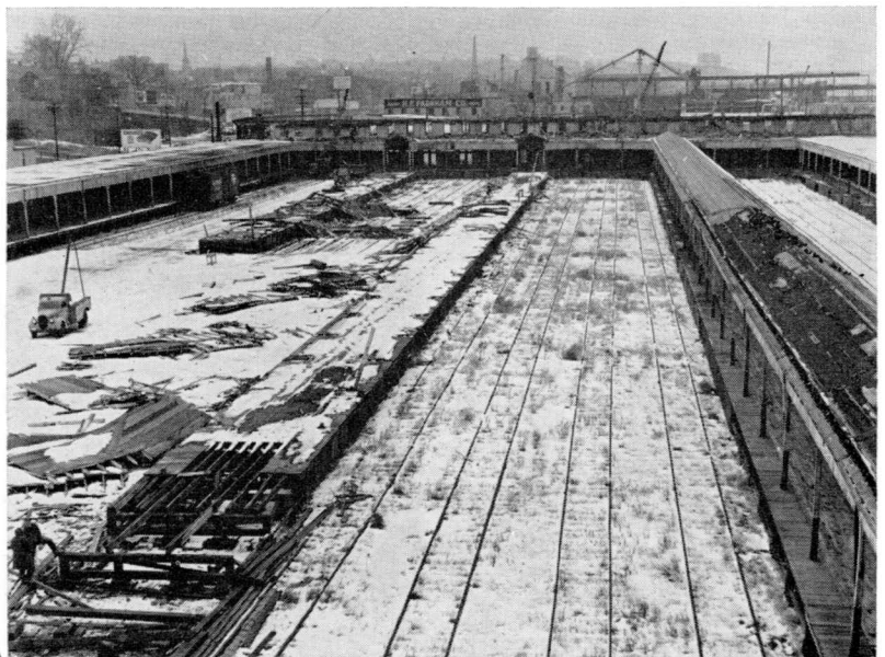
PORTLAND FREIGHT SHEDS DISAPPEARING —More than four and a half acres of land on Commercial street, Portland, will be available for industrial use when demolition of the old Portland freight house is complete. Portland Terminal Company freight office operations have been moved to Rigby.
