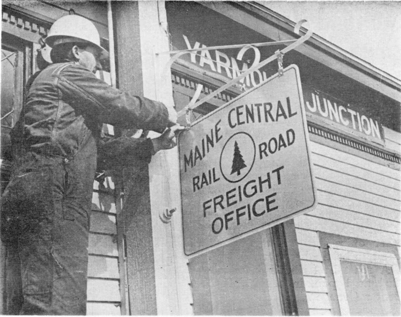
SIGN OF SPRING —On March 21, the first day of Spring, Bridge and Building crews began to install new reflectorized signs on Maine Central station buildings throughout the system designating them as freight offices. Signs are going up on the buildings themselves, like this one at Yarmouth Junction, and on posts at the ends of streets and drives that lead to the offices. Installing the new sign above is Ernest E. Henry, Waterville, B&B carpenter.
