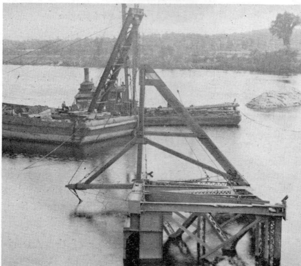
The bridge sections were rolled upright with the aid of this frame device, and with big winches on the lighters.
