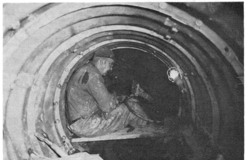
REINFORCEMENT —Putting a modern steel lining inside a stone culvert, which was originally built in the 1800's is D. A. Pomeroy, foreman of the Stone Crew. The culvert is at milepost 8 in West Falmouth. The day after the job was completed, the new culvert was filled by the Spring runoff.
