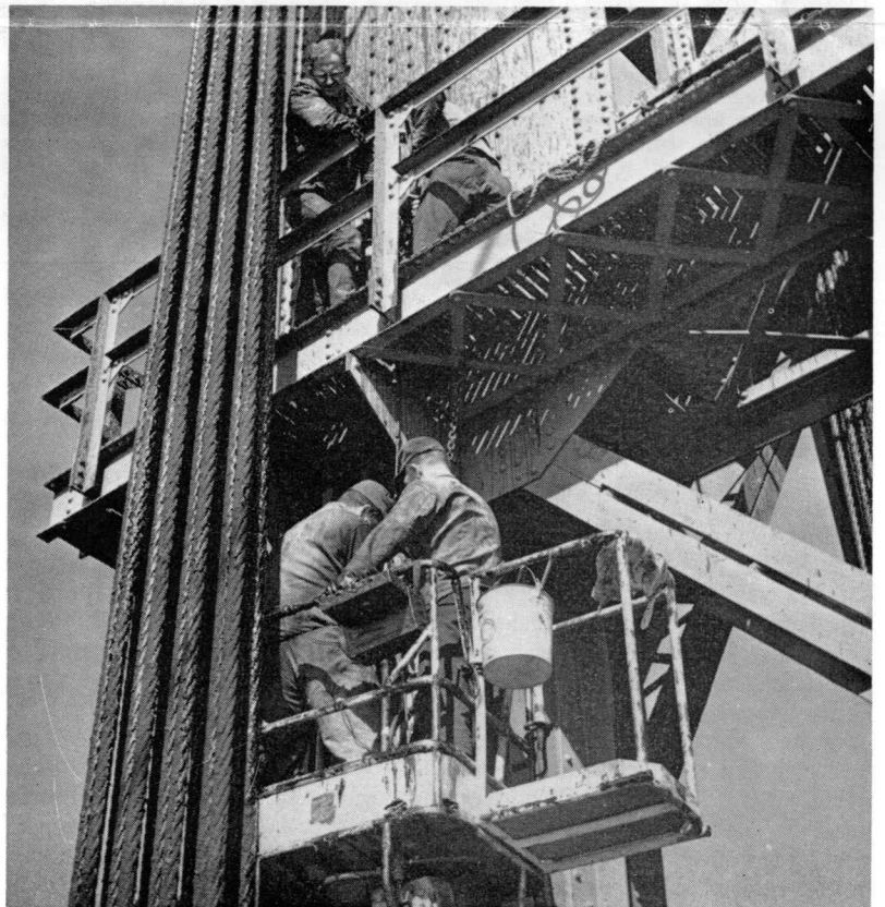
Bridge and Building crewmen install bridge lifting cable at Carlton Bridge, Bath. The photo was taken from the drawbridge deck approximately 200 feet above the water level. Crewmen are installing pin which holds cable to top of the tower. Large cables to the left are counterweight cables. Four cables were changed at this location in recent months. Work was performed by W. L. Morang's carpenter crew and R. R. Grant's paint crew, working under the direction of B&B Supervisor J. E. Lancaster. In the picture, upper left, John Kaine, Vanceboro, carpenter; right Lawrence Parlin, Augusta, painter; lower left, Foreman Ralph Grant, Portland and lower right, Lionelle Morrissette, Winslow, truck driver.
