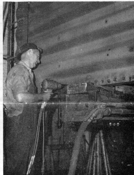
Richard Ladd, Carman Helper, uses new lock bolt machine to secure end sheet to end sill.
