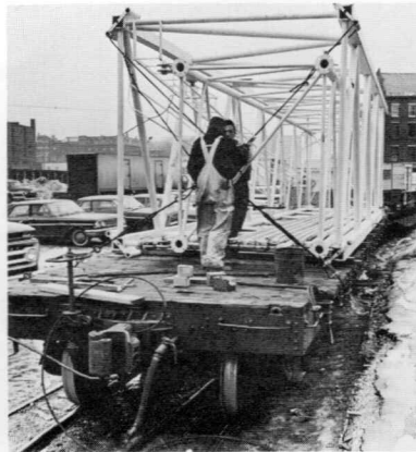
Part of the crane's boom is secured to the MeC car by longshoremen for the trip to destination.
