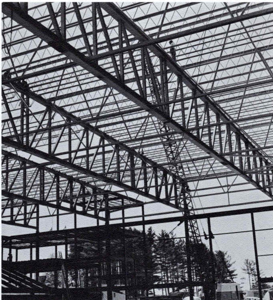
The Augusta Civic Center with most of the roof beams in place. The building is one of the largest clear span buildings east of the Mississippi. Sheridan Corp. is a major sub-contractor for the project.
