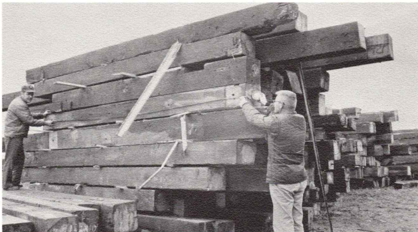
The landmark Grand Trunk grain elevator is being torn down. One million board feet of lumber from the grain elevator was transported to Rockland by Maine Central to be used in the construction of a new resort hotel. The facility will be constructed on the site of the former Samoset Hotel which burned recently. The Samoset was once owned by the Maine Central.
