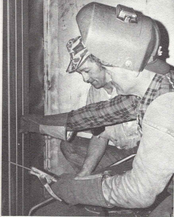
Waterville Shop workers, carman welder Aurele Michaud, right, and carman Edward King install steel end lining in a boxcar rebuilt at the Shops with incentive per diem funds.
