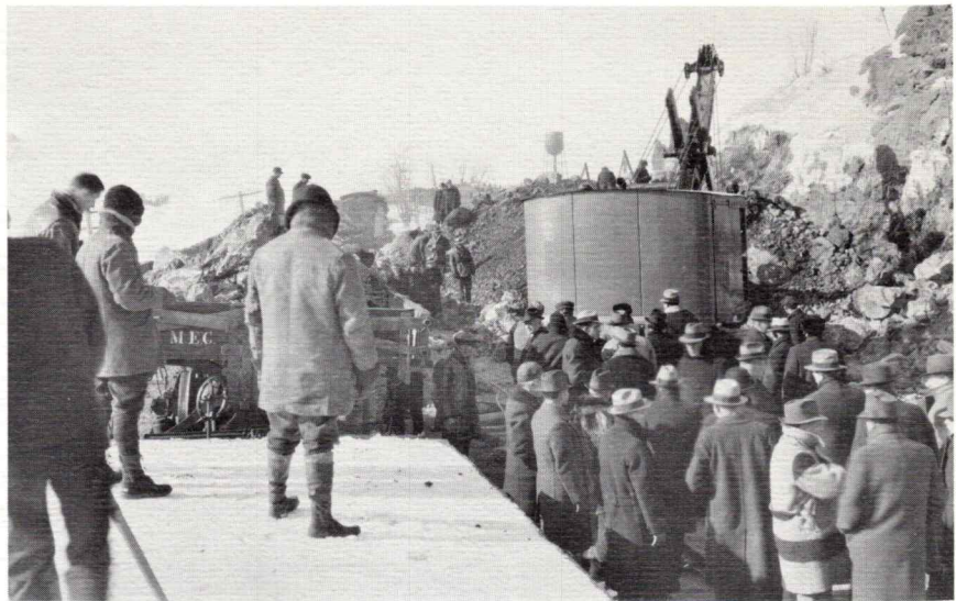
Maine Central crews are shown loading rocks into railroad cars on a cold February 7, 1936. Many Eastport dignitaries were on hand for the first day of the operation. The location is near Carrying Place Cove on the Emery property. It was after this work was completed that Eastport was no longer an island, but joined to the mainland by the first step of the Quoddy project. Photo from Will Beale collection.
