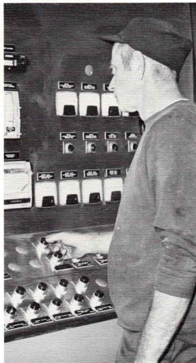
A Pejepscot Paper employee makes some last minute checks on the control board of the new mill.
