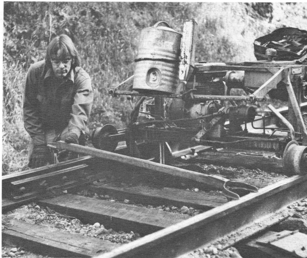
Trackman Gerry Desveaux checks track gauge immediately ahead of the tie plate placer.
