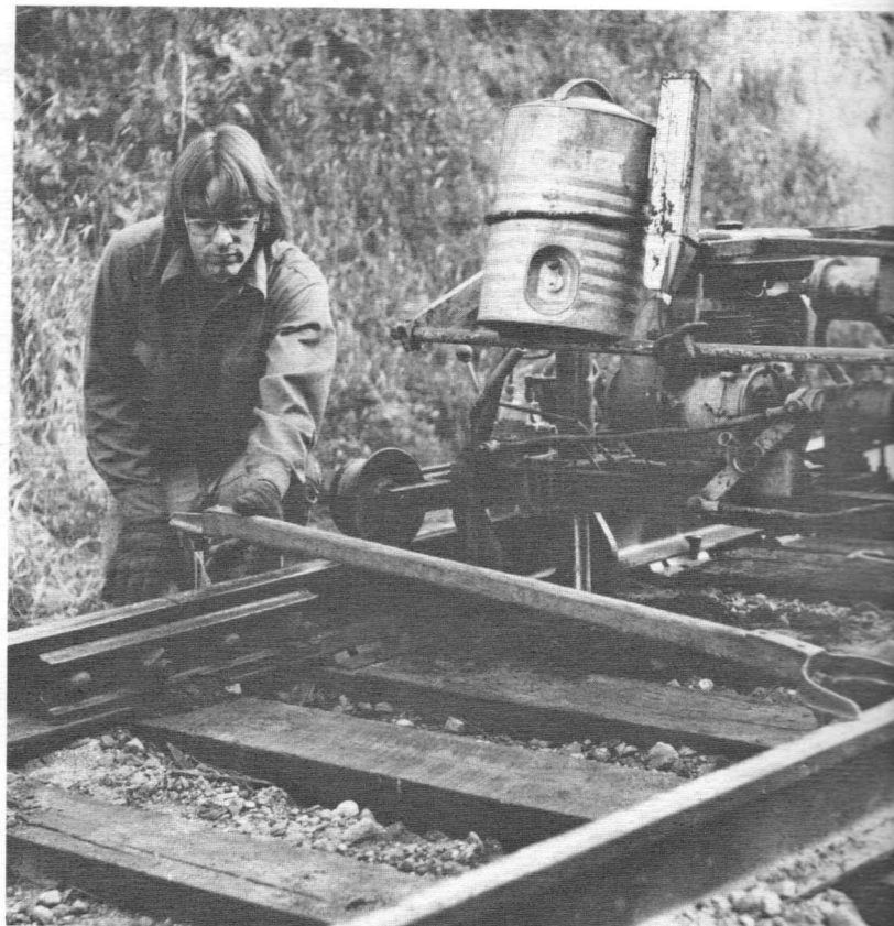
Trackman Gerry Desveaux checks track gauge immediately ahead of the tie plate placer.
