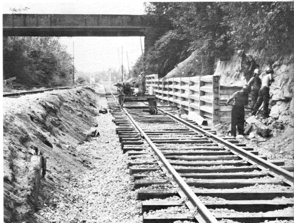
Railroad clearances have been improved by lowering the main line and side track at the Riverside Street Bridge in Lewiston. At the time this picture was taken, the side track had been lowered more than three feet. The main track was lowered a few weeks later.
