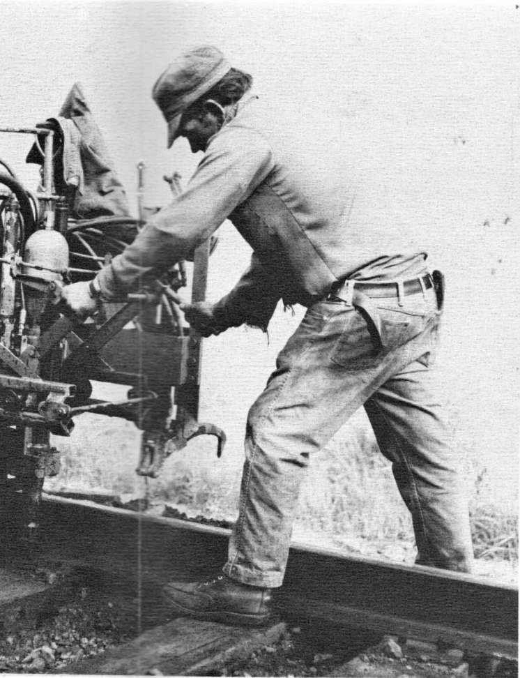
John Hunnewell is driving spikes in a new cross tie with a spike driver.
