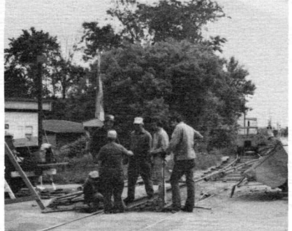
Track repairs on the Main Street crossing in Waterville by Maine Central track crews.
