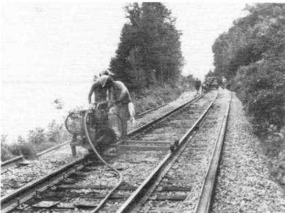
Maine Central's first continuous welded rail was installed along the shore of Messalonskee Lake, near Belgrade, in June.
