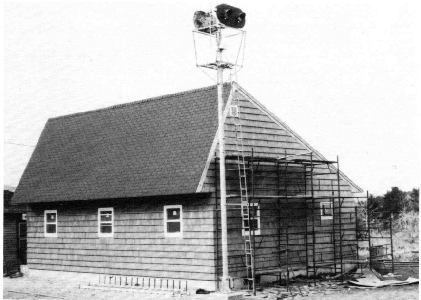
The new station at Rileys, completed last month, is just one step short of being a solar-heated prototype of a new generation of Maine Central stations. The step: how it works out next winter.
