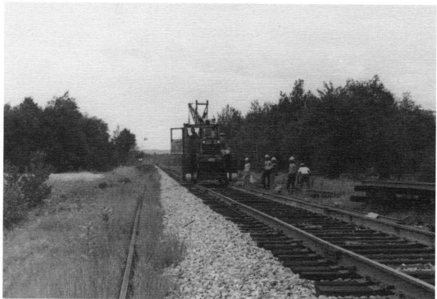
Continuous welded rail was installed this summer in four miles of main line at New Gloucester. Crews are shown as they finished spiking the far rail, just before placing and installing the near rail, shown in the grass at the left of the roadbed. This area is just above the Route 231 crossing, looking toward Danville Junction.
