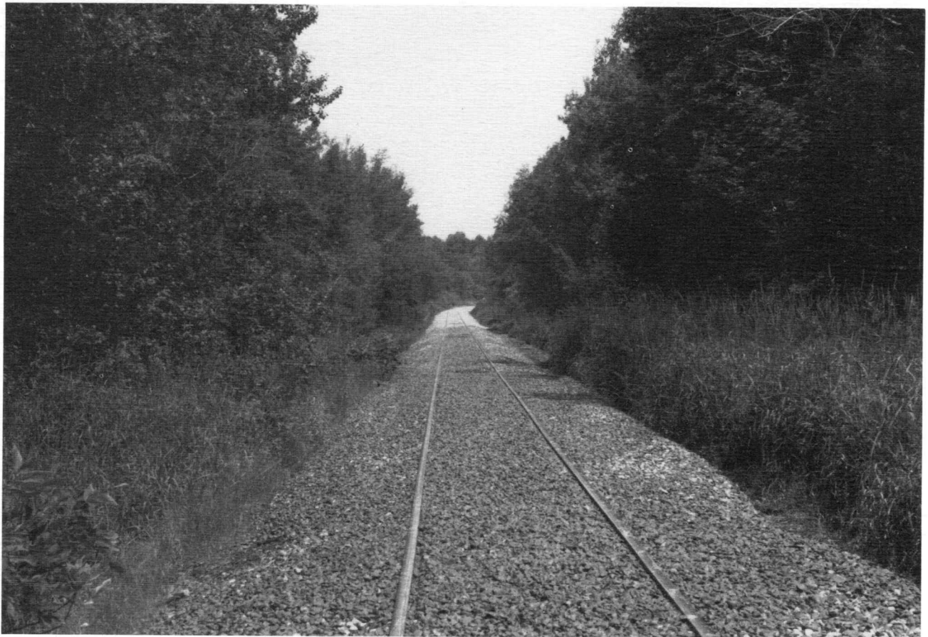
With ballast in place and ready for the tamper, this section of the Bucksport Branch is smooth and straight and improved for heavier loads of freight from industries at Bucksport and Orrington.
