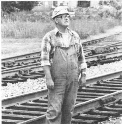
Lawrence T. Caret, leading signal maintainer, Waterville, watches his crew repair a crossing signal.
