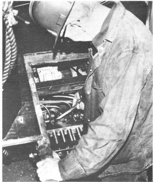
Piper Bill Brown piping to air brake modular system manifold.
